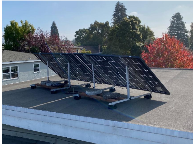
Plug-in solar system installed on a rooftop in Berkeley, CA. Photo Credit: CESA.
