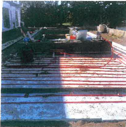
Spa in slab heating system
