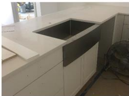
Unit kitchen sink
